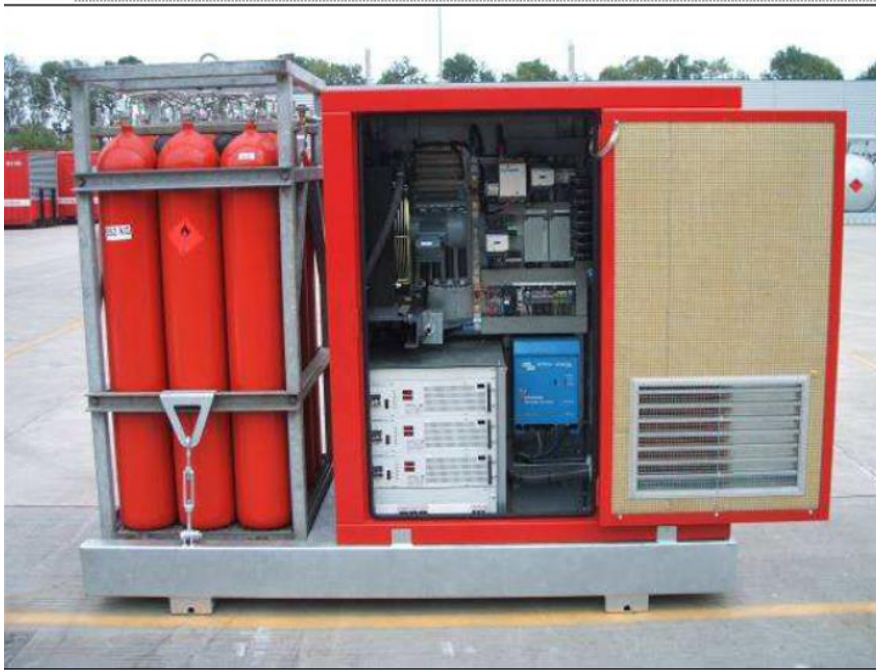
Electric Side of the Canopy
